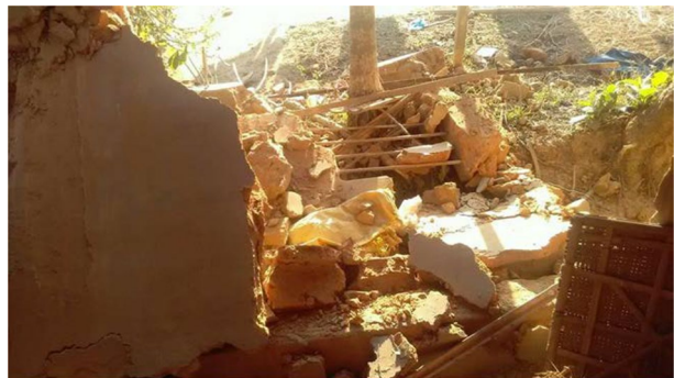
Fig. 16 Out-of-plane failure at one of the mud houses in Tripura
