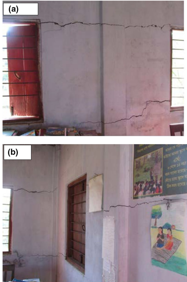
Fig. 12 a, b Damage caused to a masonry building with light GI (galvanized iron) sheet roofing which lacks lintel band
